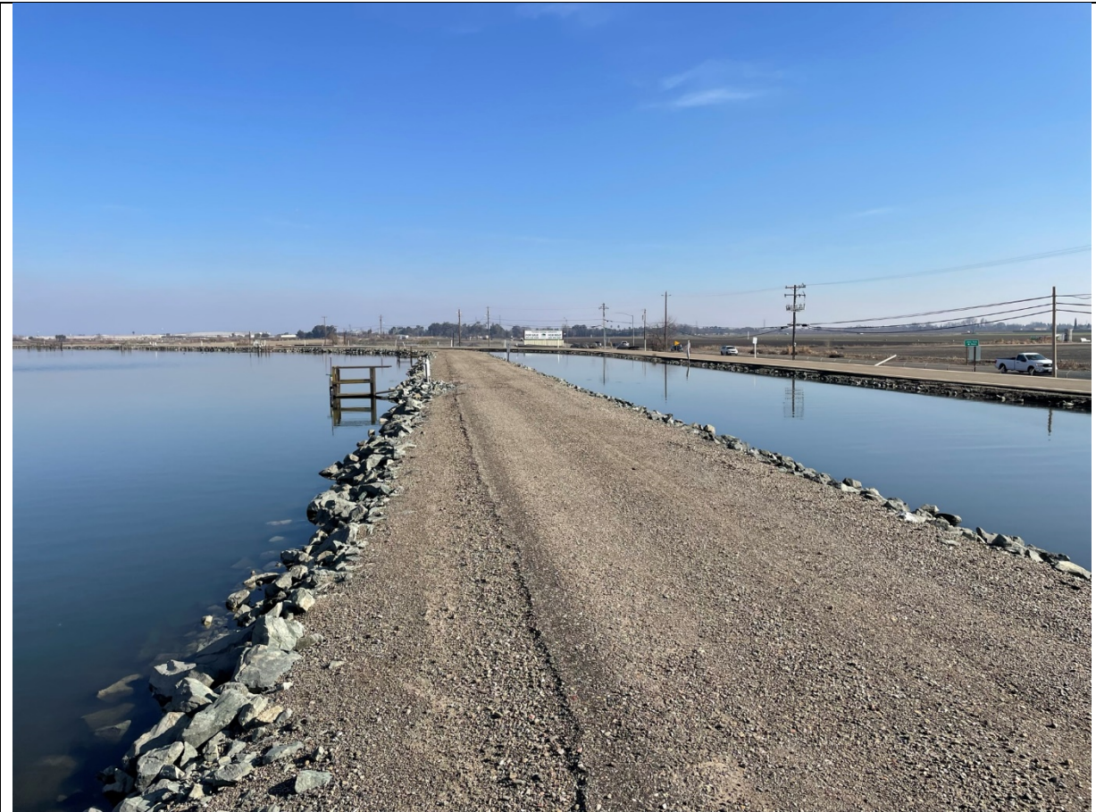
Photo 5: View looking east near B-3. Loose gravel exposed from surface layer of asphalt deteriorating.
